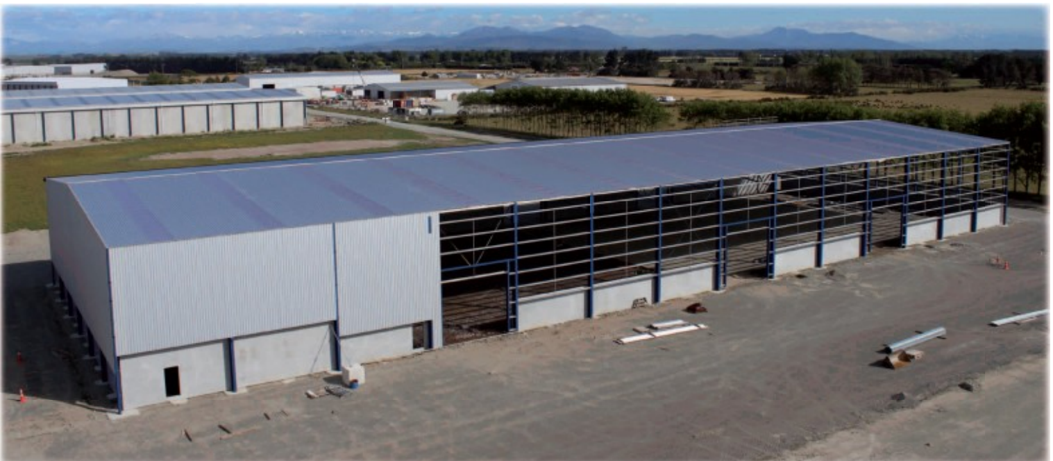
Roof on, wall cladding in construction and floor set out for concrete pour
